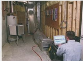
Inside job. Aero-seal uses a process in which a nontoxic mist is sprayed inside the home's ductwork system. The company says that the aerosol finds and seals even the most inaccessible leaks.
