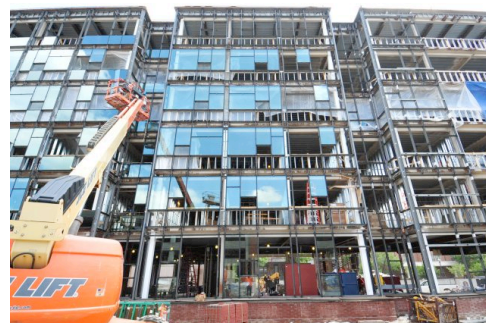
Construction of William Hall Complex Expansion on schedule and ready to open in Fall of 2012
