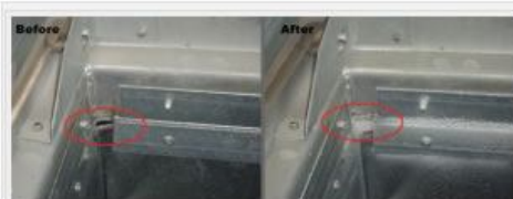
Sealant particles do not coat the entire inside of the shafts but form a tight seal around individual leaks. PHOTO: Aero Seal LLC and Steven Winter Associates Inc.
